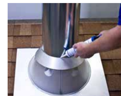
13. Apply high temperature silicone sealant where storm collar will meet chimney. Slip storm collar around chimney and slide down. Seal with high temperature silicone sealant.
