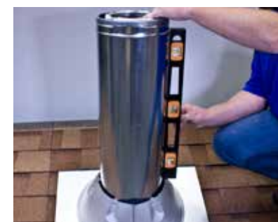
12. Add more chimney sections until chimney is at least 3 ft above roof, and at least 2 ft above any part of your house within 10 ft.
